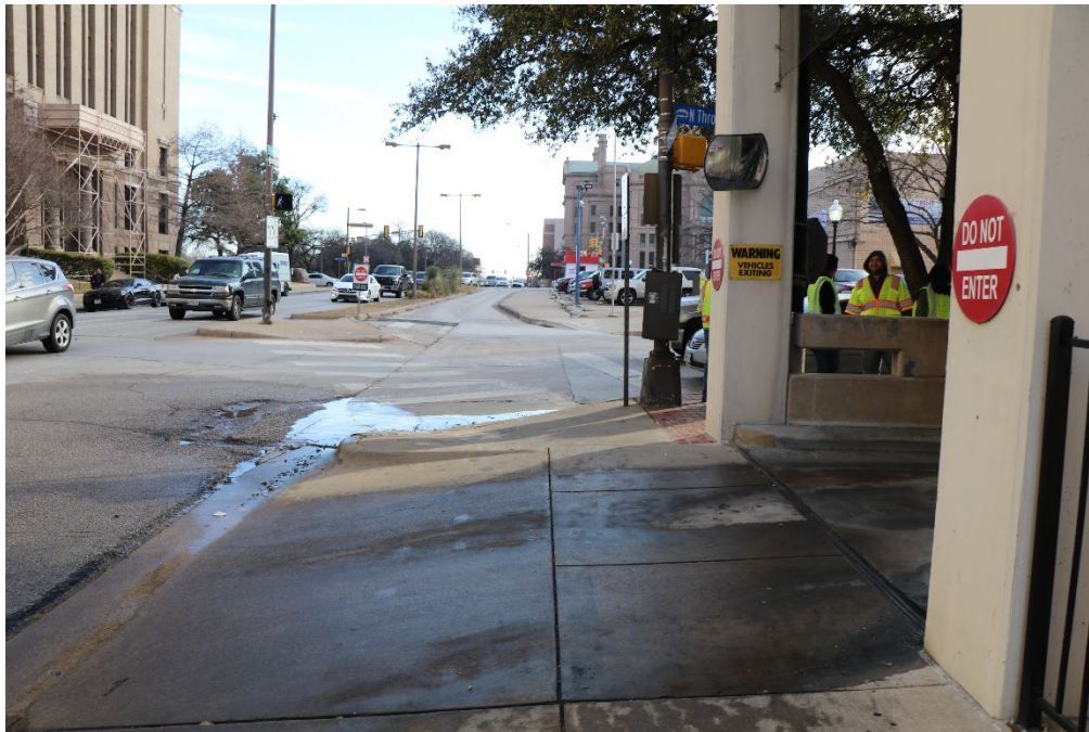
Figure 11: Misaligned crosswalks and ramps at Throckmorton Street, with bus/bicycle turnaround
