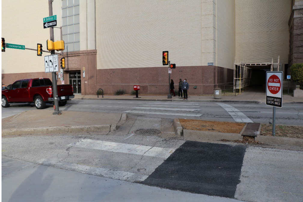
Figure 12: Misaligned crosswalks and ramps at Throckmorton Street
