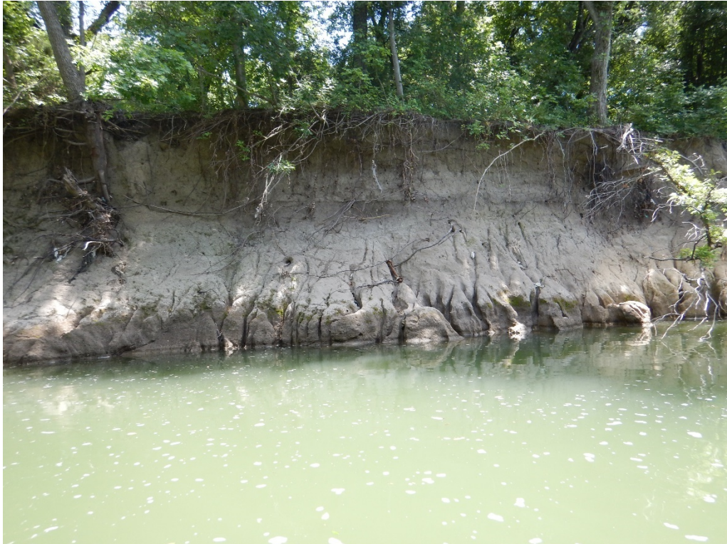
Rowlett Creek in Garland on June 18, 2020. Photo faces the right bank at transect 5 and illustrates severe ongoing bank erosion with near vertical banks.
