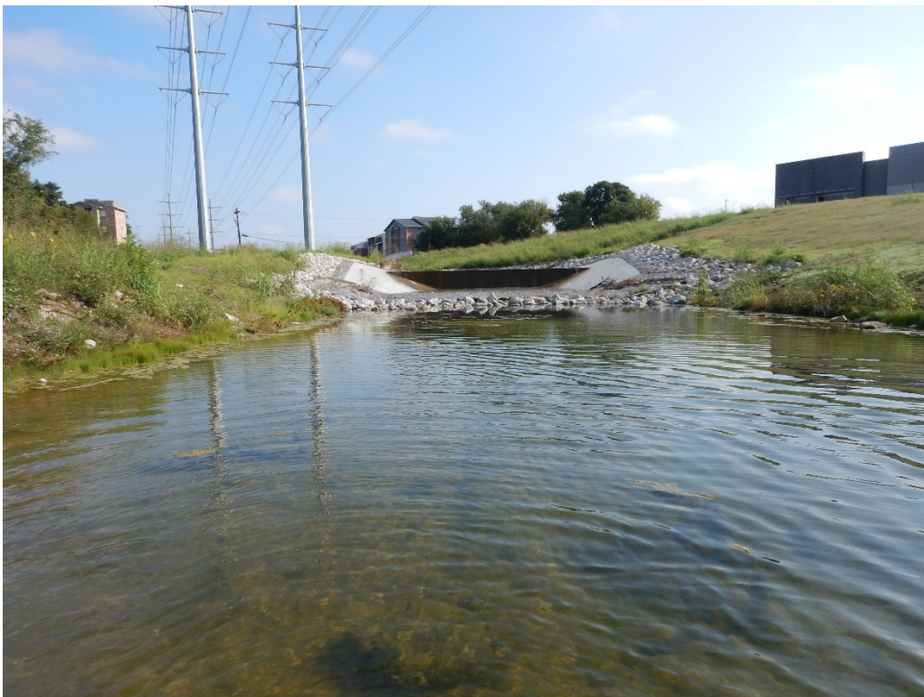
Estelle Creek in Irving on September 25, 2020. Photo faces upstream from habitat transect 3 and illustrates one of the low head dam structures within the assessment reach.
