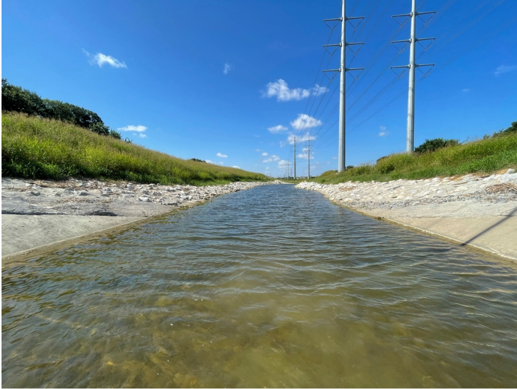
Estelle Creek in Irving on June 24, 2021. Photo faces downstream from habitat transect 5 and illustrates a long pool/glide habitat with concrete lined banks.
