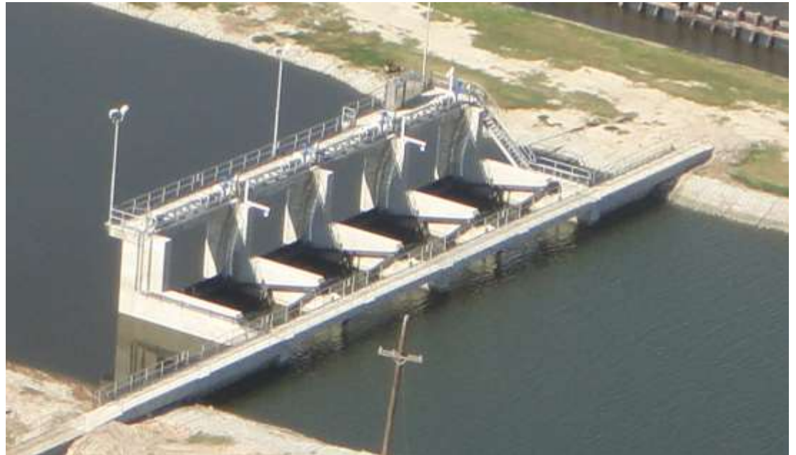
4-gate combination salt-water barrier and flood conveyance structure , Taylor Bayou near Gulf Intracoastal Waterway
